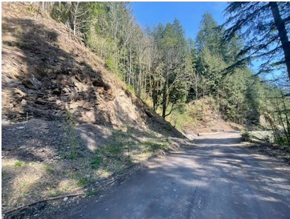
Approach from town, unstable slope above
