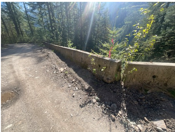
Road material scours down
