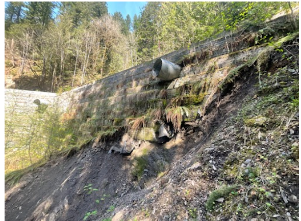
Woods culvert outlet. Failed wall below culvert. Seepage below culvert evident.
