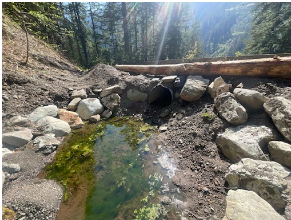
Town culvert inlet high.
